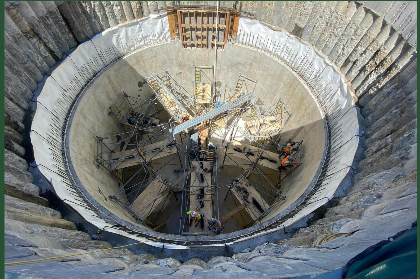
BP1 Wet Well, April 2022
