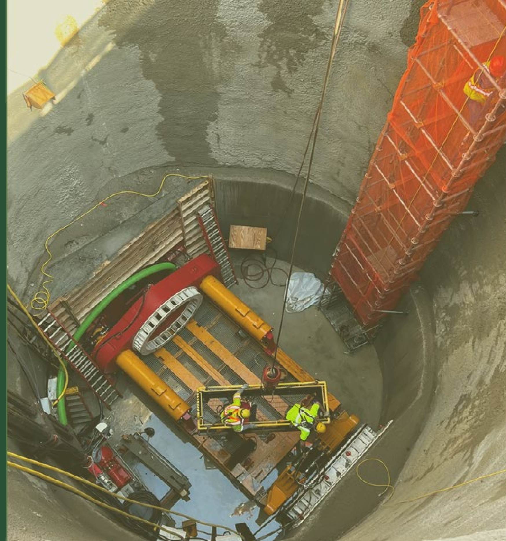
Jacking Station for Microtunnel Boring Machine (MTBM) named MARSH-MELLOW at Bay Park Shaft 2, March 2022
