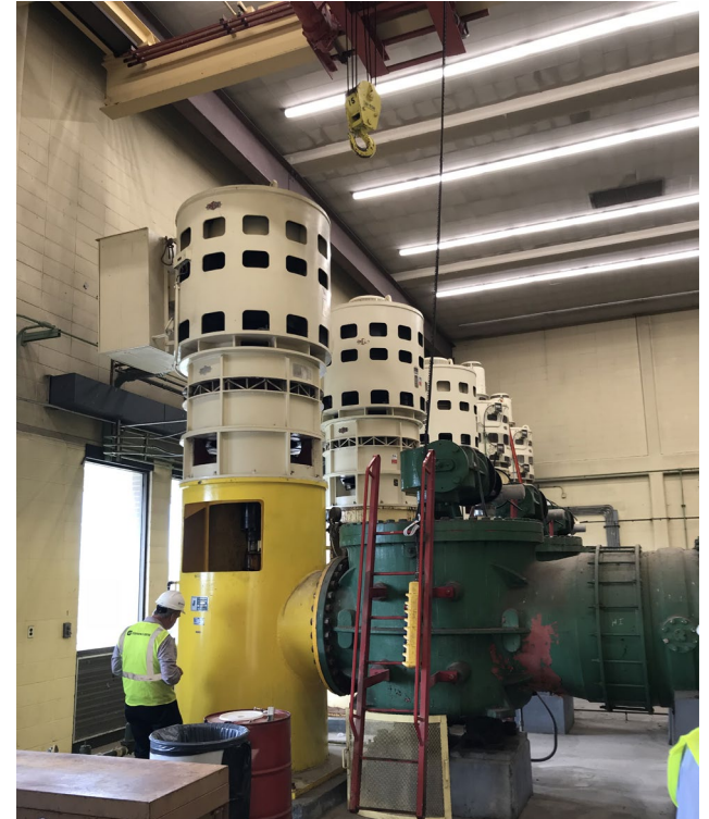
Cedar Creek, existing tide pumps
