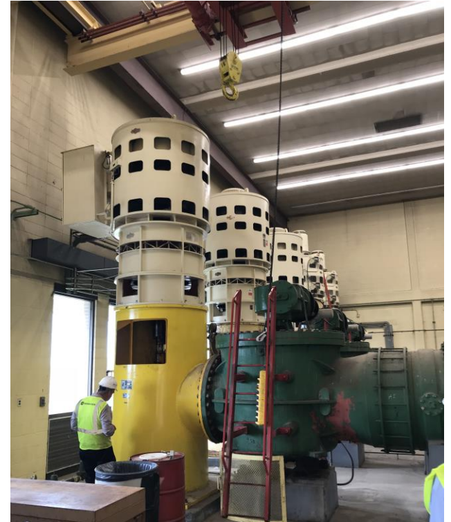
Cedar Creek, existing tide pumps
