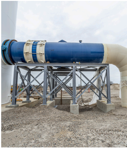
Pipeline from Receiving Tank
